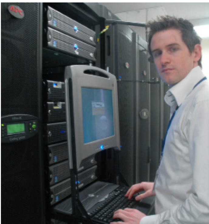
Technology Analyst Michael Coyne in the new datacentre
