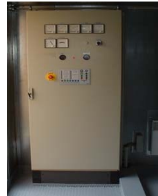
Generator regulation and distribution
