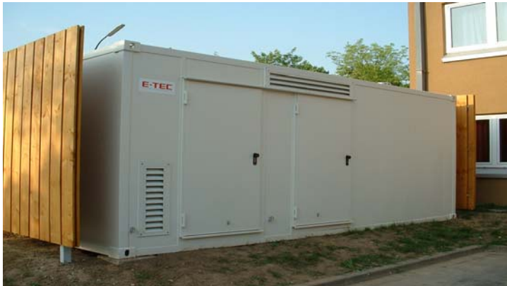
20 feet Container with electrical operating room for UPS +Generator
